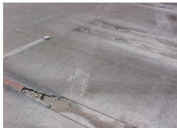
Figure 1: Crack and Spall
